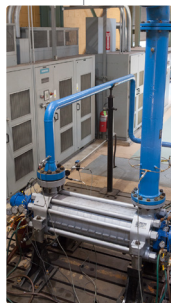
CERTIFIED PERFORMANCE TESTING
