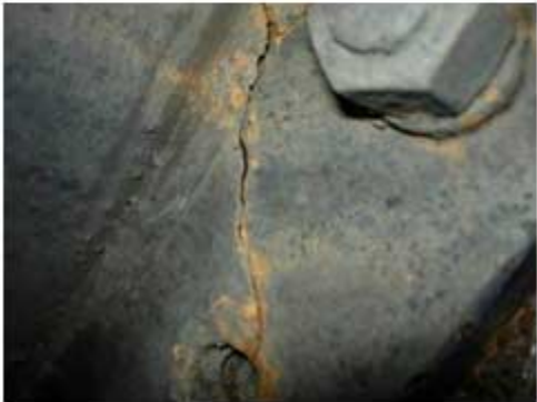
Close-up of the broken pipe flange
