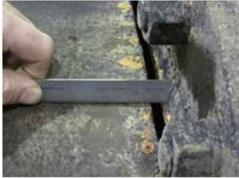
Close-up of the broken pipe
