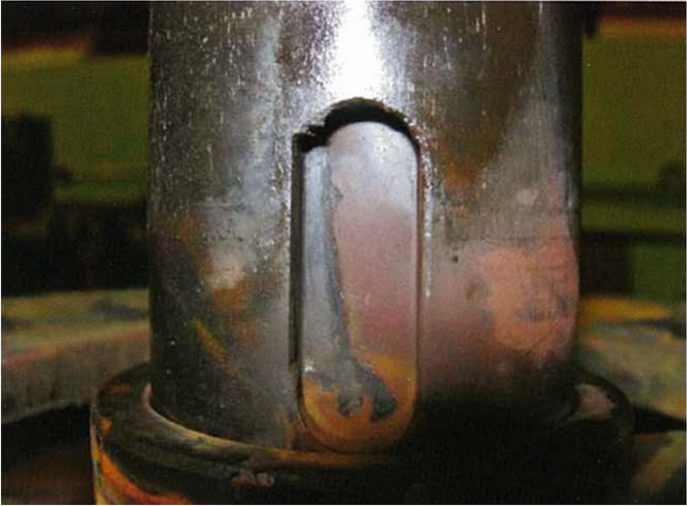
Deformed keyway on pump shaft
